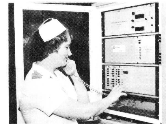
Sr. Merryl Owen, Corio House, testing the fire control board with the Country Fire Authority.
