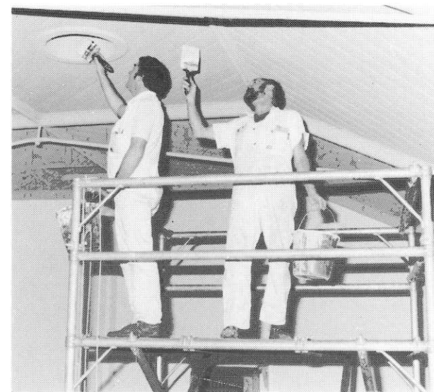
Painters Ron Johnston and David Stocks repaint the ceiling of the community service block during its conversion to the new Physiotherapy Dept.
