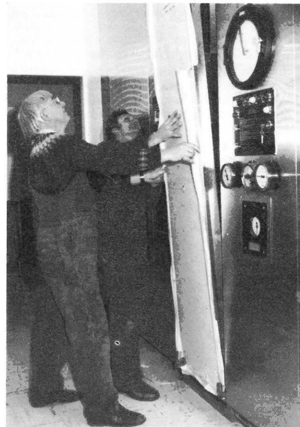
Hospital maintenance staff Mr. John Lyons and Mr. Tom Lucas complete the installation of a new Hi-Prevac sterilizer in the Central Sterile Supply Department.
