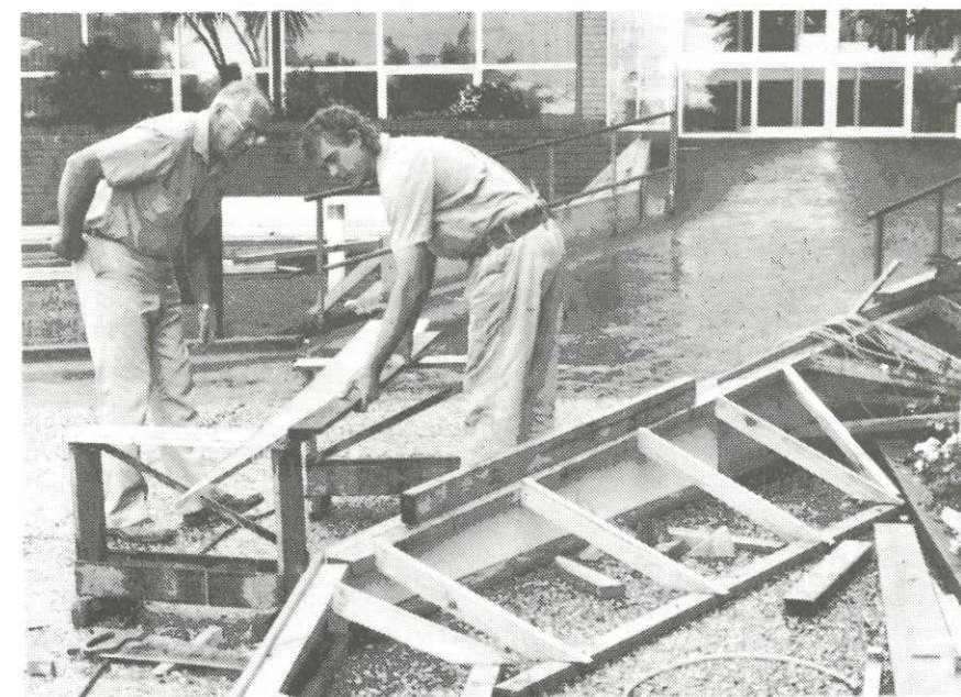
• Carpentry staff constructing the framework for the new access ramp to the main Hospital entrance.
