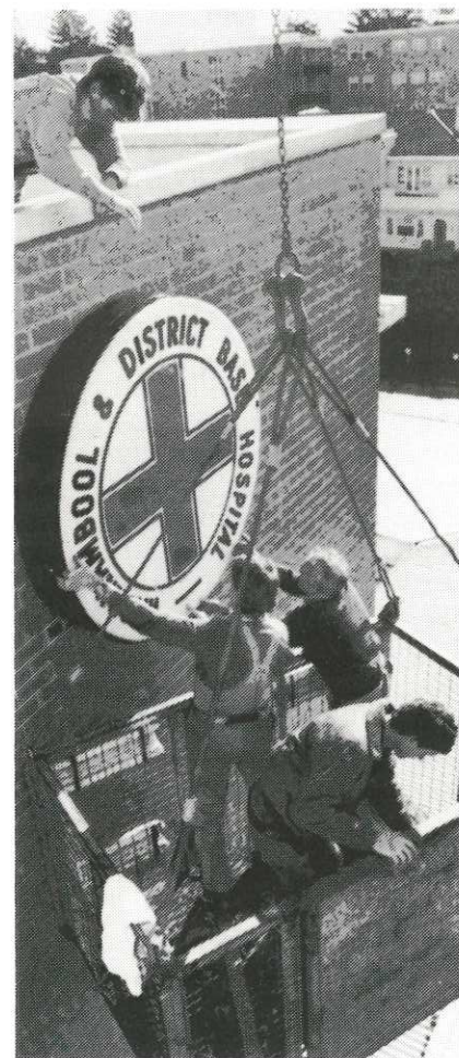
• The electricians use a crane cage to reach the illuminated Hospital logo on the multi-storey block. The Hospital's size and function often dictates the way maintenance work must be done.
